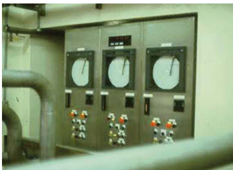
Figure 8.4 Temperature control panel
