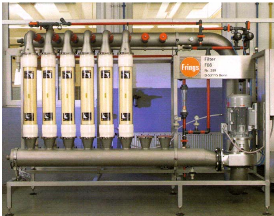
Figure 6.13 Fully automatic tangential flow filtration plant (courtesy of Heinrich Frings)
